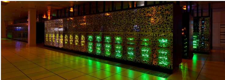
The CURIE supercomputer installed at TGCC
